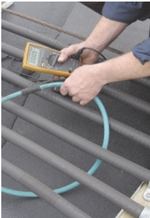
The built-in pulsing circuit alters the fault current, creating a two-stage pulse that can be traced using a handheld meter and current sensor to quickly locate a fault.
