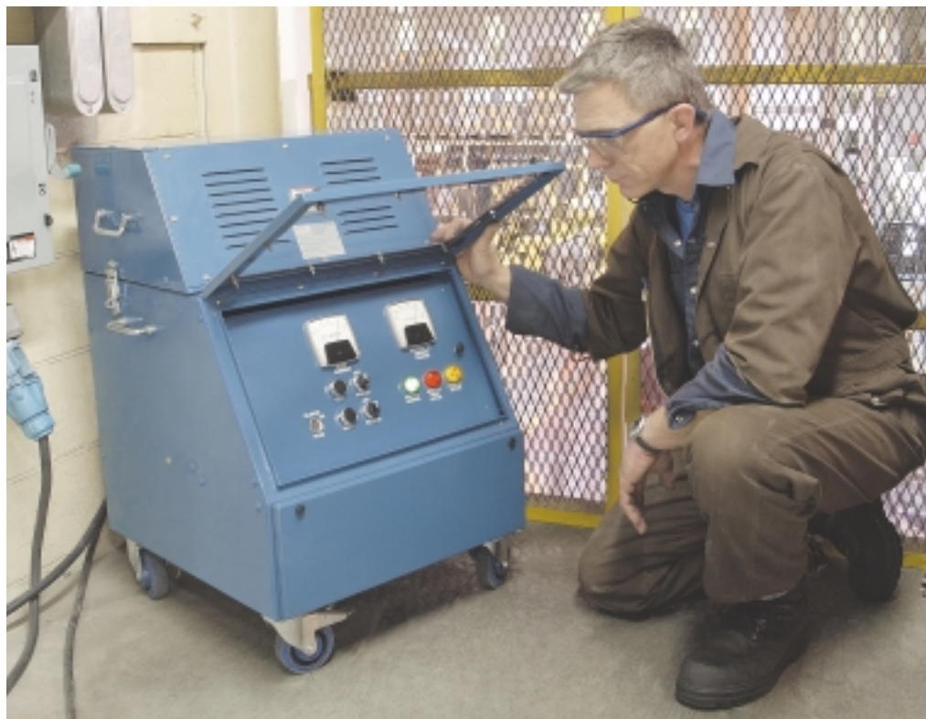
Vic Galamb of Collins Electric uses IPC's portable pulsing ground fault detection system to locate faults at the Narmco autoparts manufacturing facility, without disrupting production.
